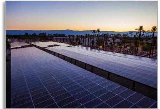
Solar Photovoltaic System
