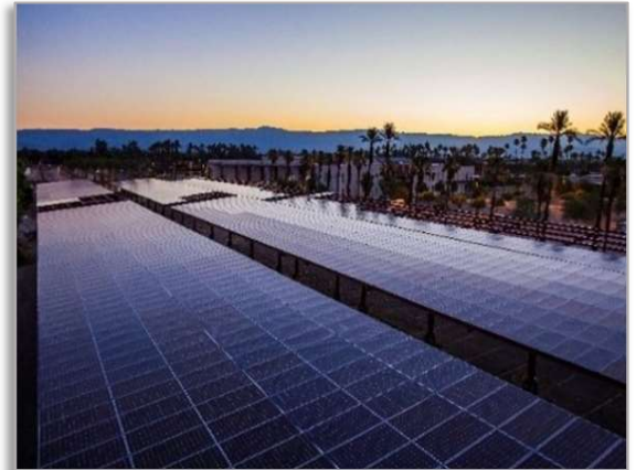
Solar Photovoltaic System
