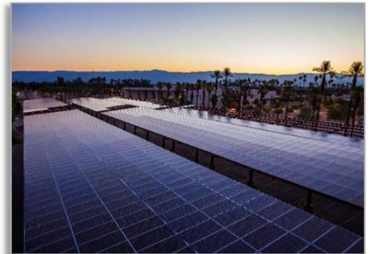
Solar Photovoltaic System
